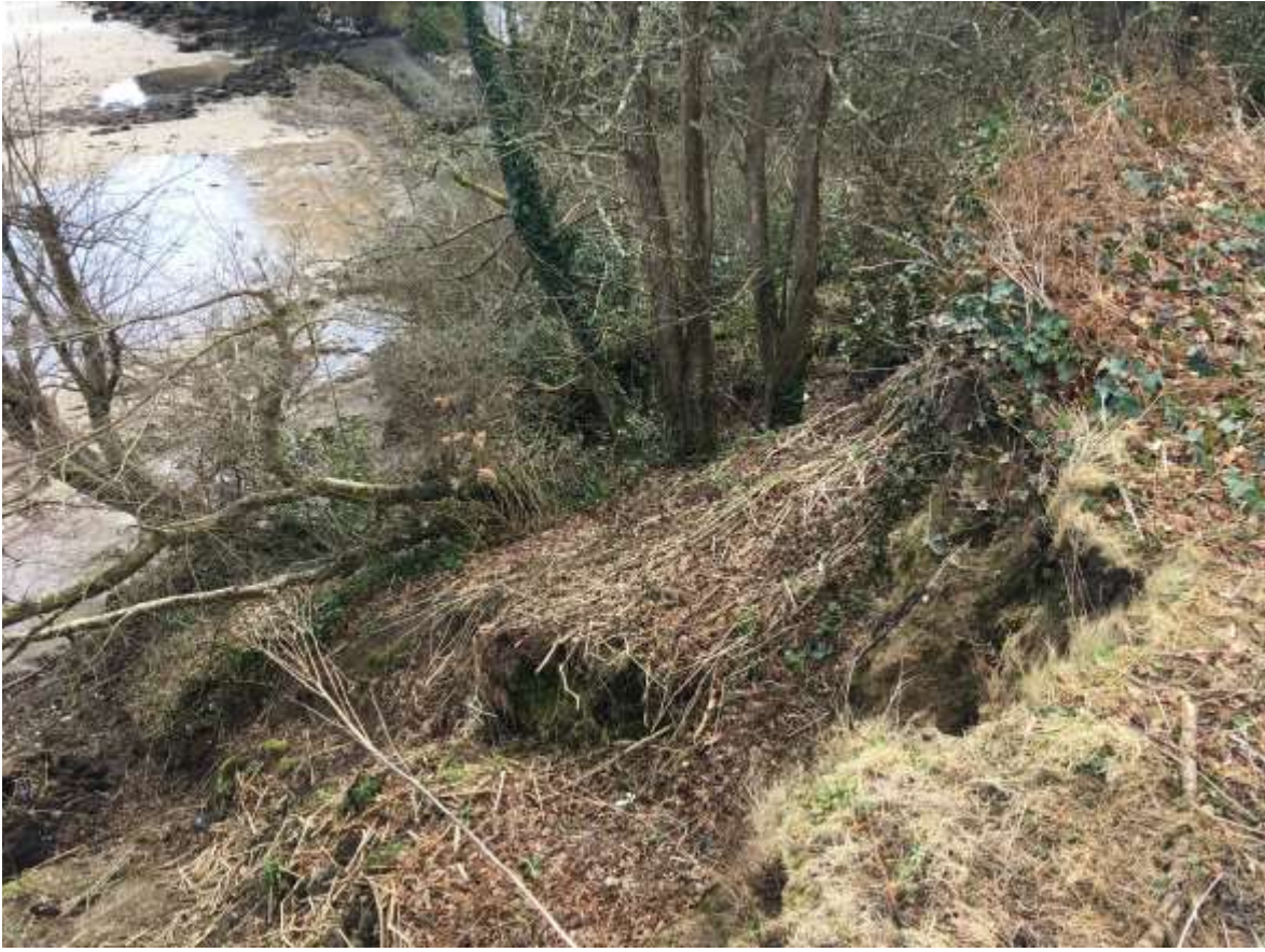
Photograph 2- Dead stems of Himalayan balsam cover the majority of the collapsed slope
