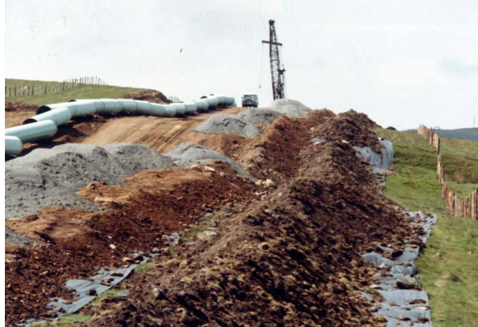
Good practice on an RML pipeline project - thin mountain soil stripped in 2 layers and separated from the undisturbed ground by a membrane to simplify restoration work along the 'right of way'
