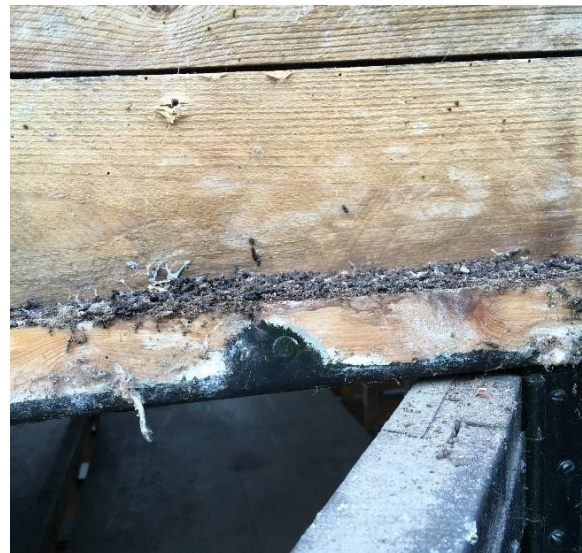
Accumulation of bat droppings noted on ledge above door
