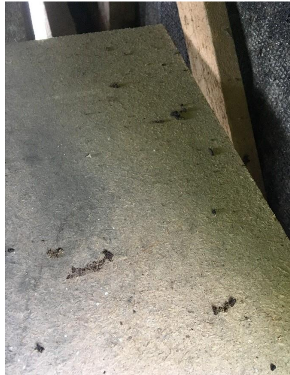
Bat droppings on crawl board in the roof space
